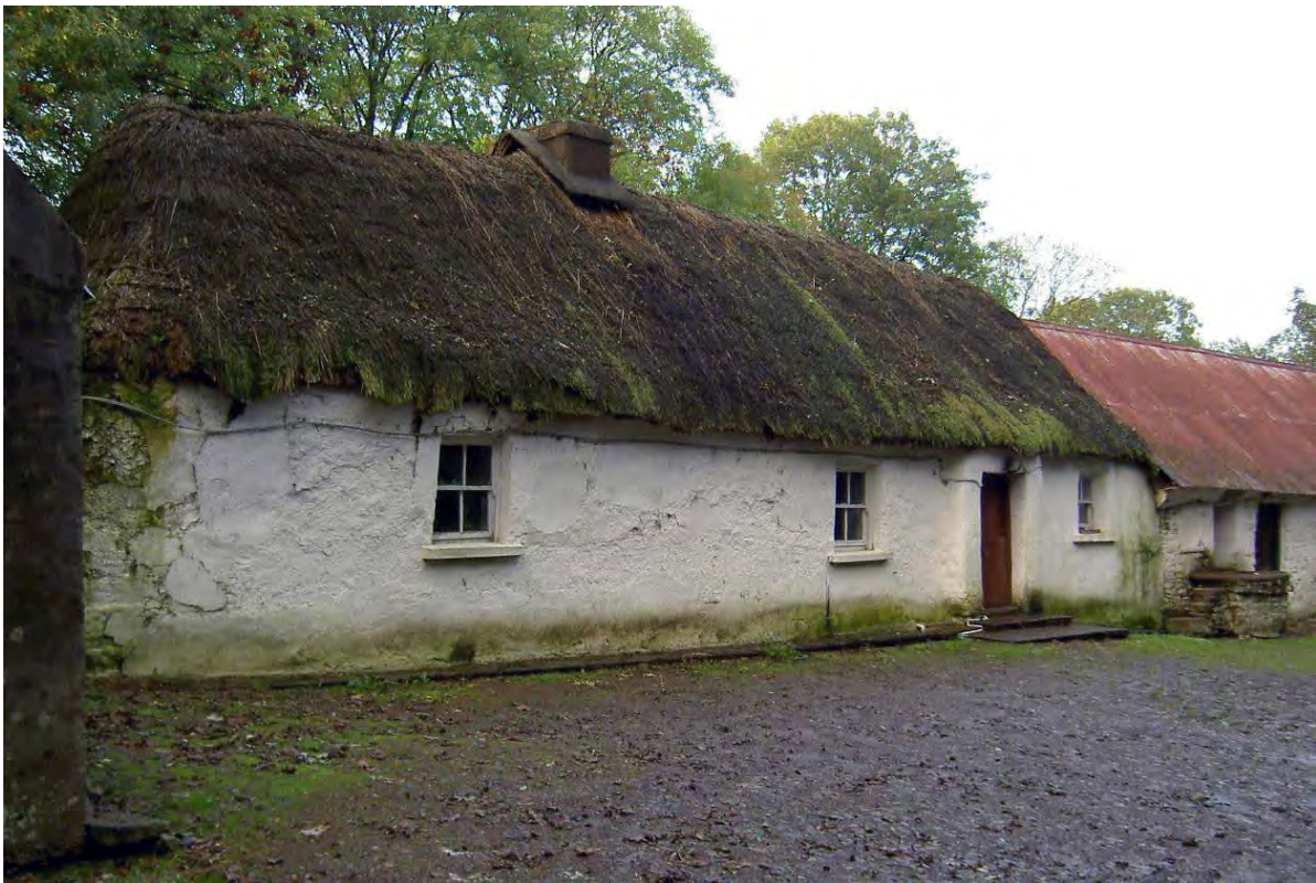
Thatched roof needing attention at Glanycummane Lower, Freemount, Co. Cork (NIAH)
