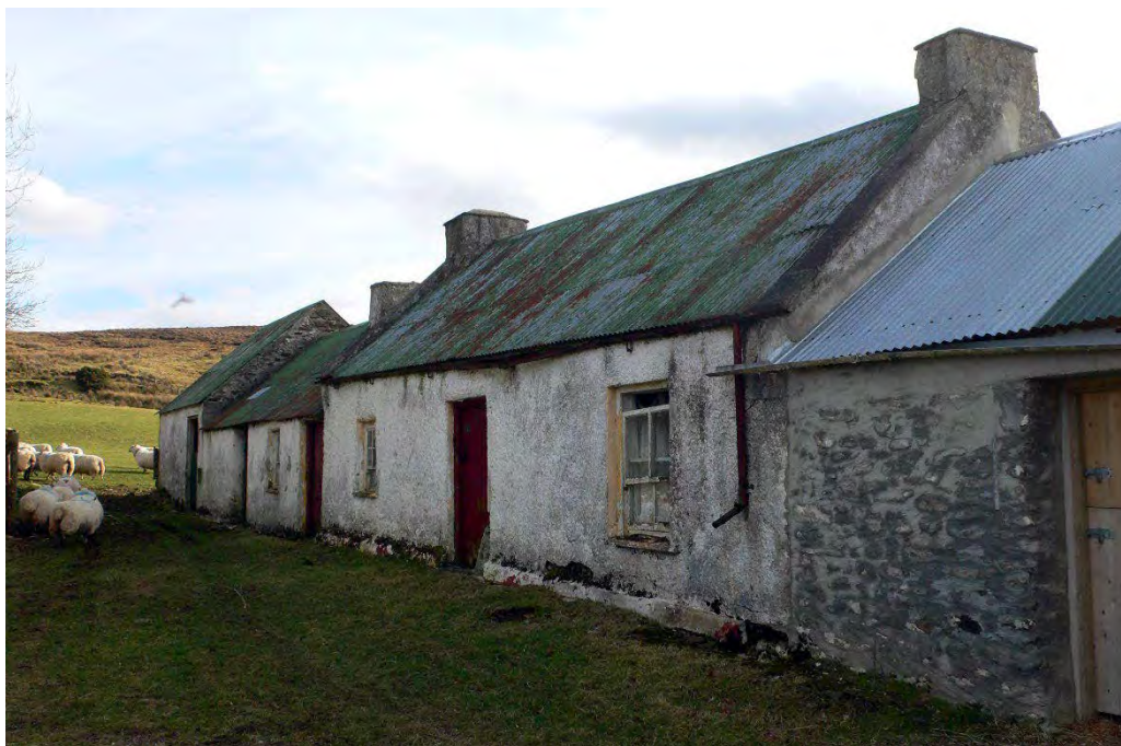
House needing repairs Cregg, near Strabane, Co. Tyrone (Barry O'Reilly)
